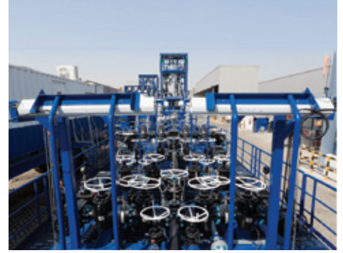
Wellhead choke manifolds and solids management trailer.
