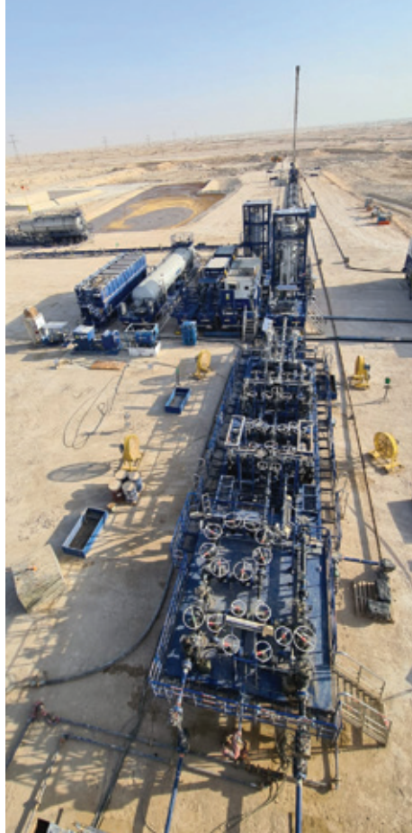
A view of the complex custom-built flowback system deployed to the operator's site within 5.2 days.
