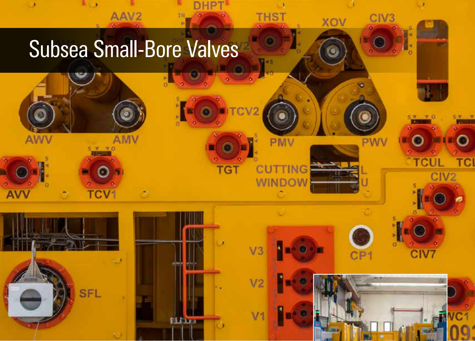
Subsea tree ROV panel with multiple small-bore valve ROV interfaces.
